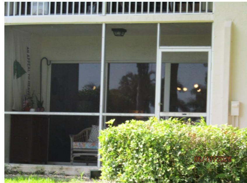
Unprotected Glazed Entry Door
