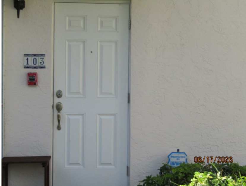
Unprotected Solid Entry Door
