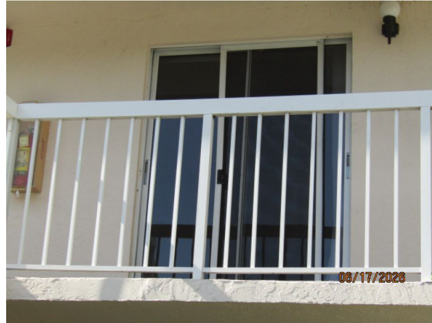
Unprotected Glazed Entry Door
