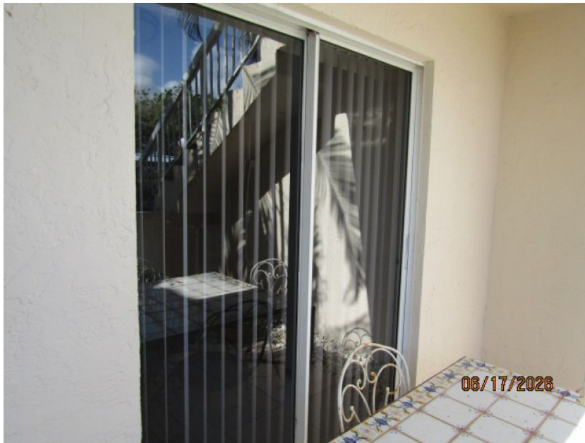
Unprotected Glazed Entry Door
