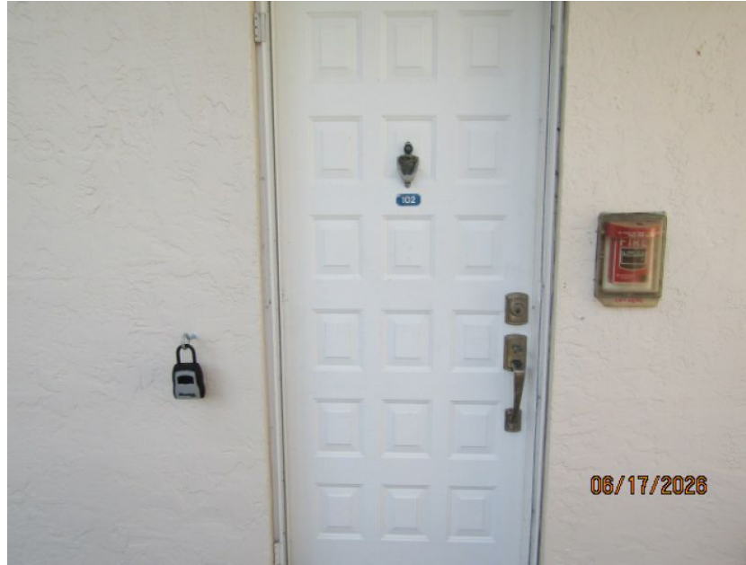
Unprotected Solid Entry Door
